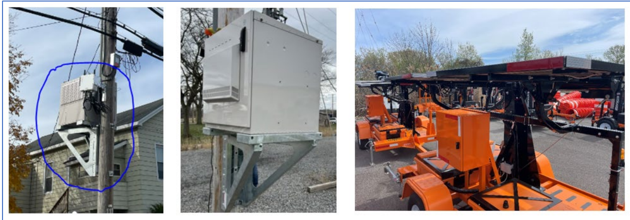
Figure 2.4: Pole Mounted extended battery backup solution and mobile connecting grid router
