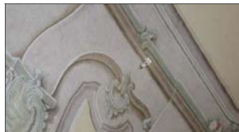
Water sprinkler installation, Schonbrunn Palace, Vienna
